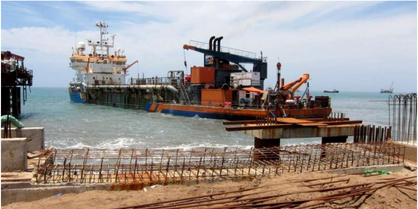
The HAM 312 seen dredging in front of jetty in Kattupalli India – Photo : Hans van Boeschoten (c)
